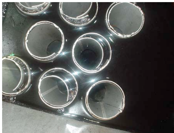
C1 EFFECT PARTIALLY COLLAPSED TUBE LINERS IN INTERNAL HEATER
